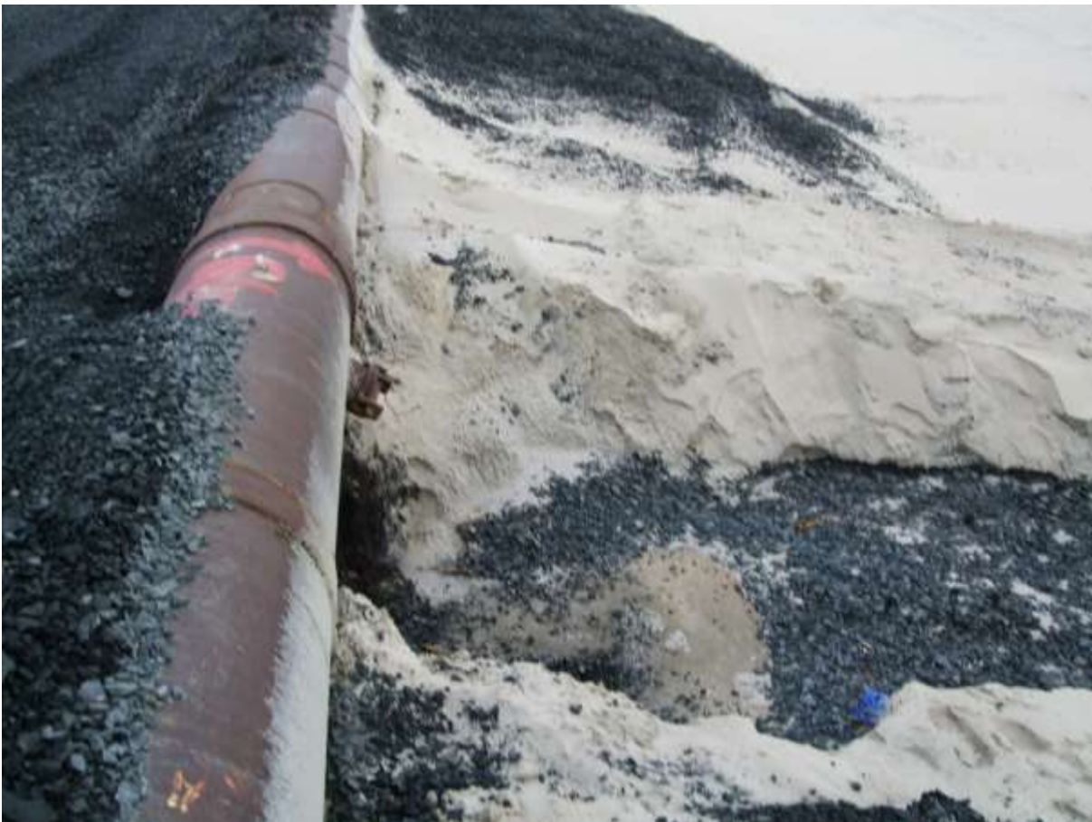
Figure A8.16: External slope of the tailings dam. The promontory arose as a result of uncontrollable surface run-off
