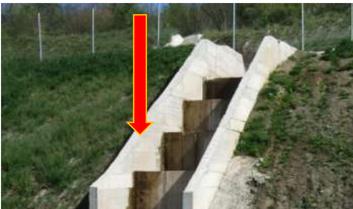
Figure A8.32: Measure 21C – Install additional drainage facilities. Drainage spillway of cascade type is installed at the tailings dam
