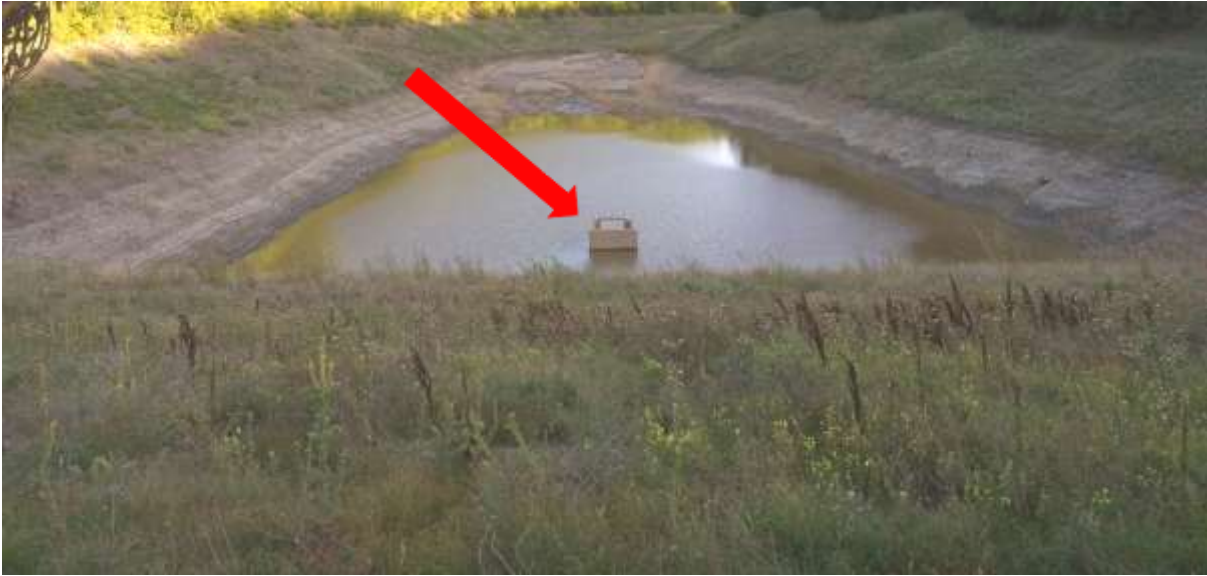
Figure A8.15: Tailings pond. The spillway remains above the water level, which can be interpreted as the implicit sign of leakages from the tailings pond due to permeable waterproofing.
