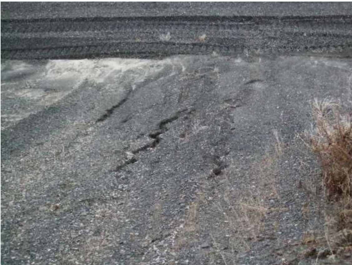
Figure A8.18: External slope of the tailings dam. Small gullies that may become ravines.
