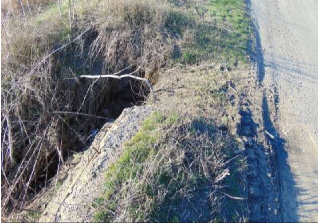
Figure A8.17: External slope of the tailings dam. The promontory appeared as a result of uncontrollable flow of precipitation water
