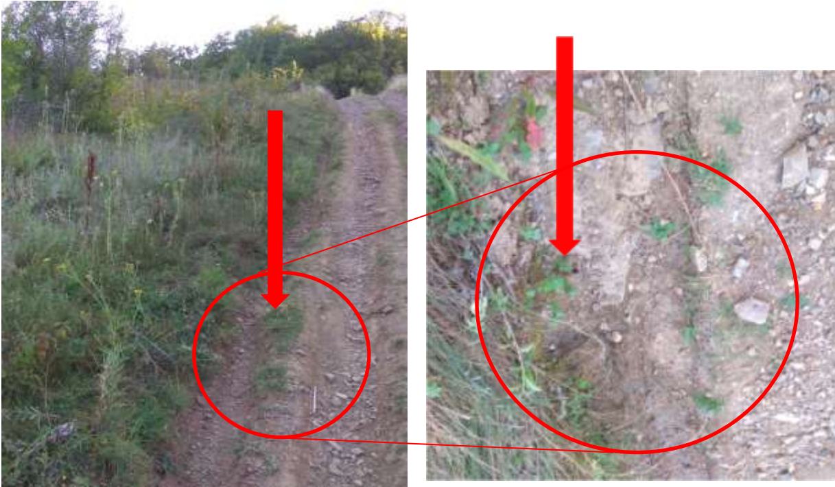
Figure A8.11: Central part of the external slope of the tailings dam. Seepage is identified in the form of spots of soil moisturizing
