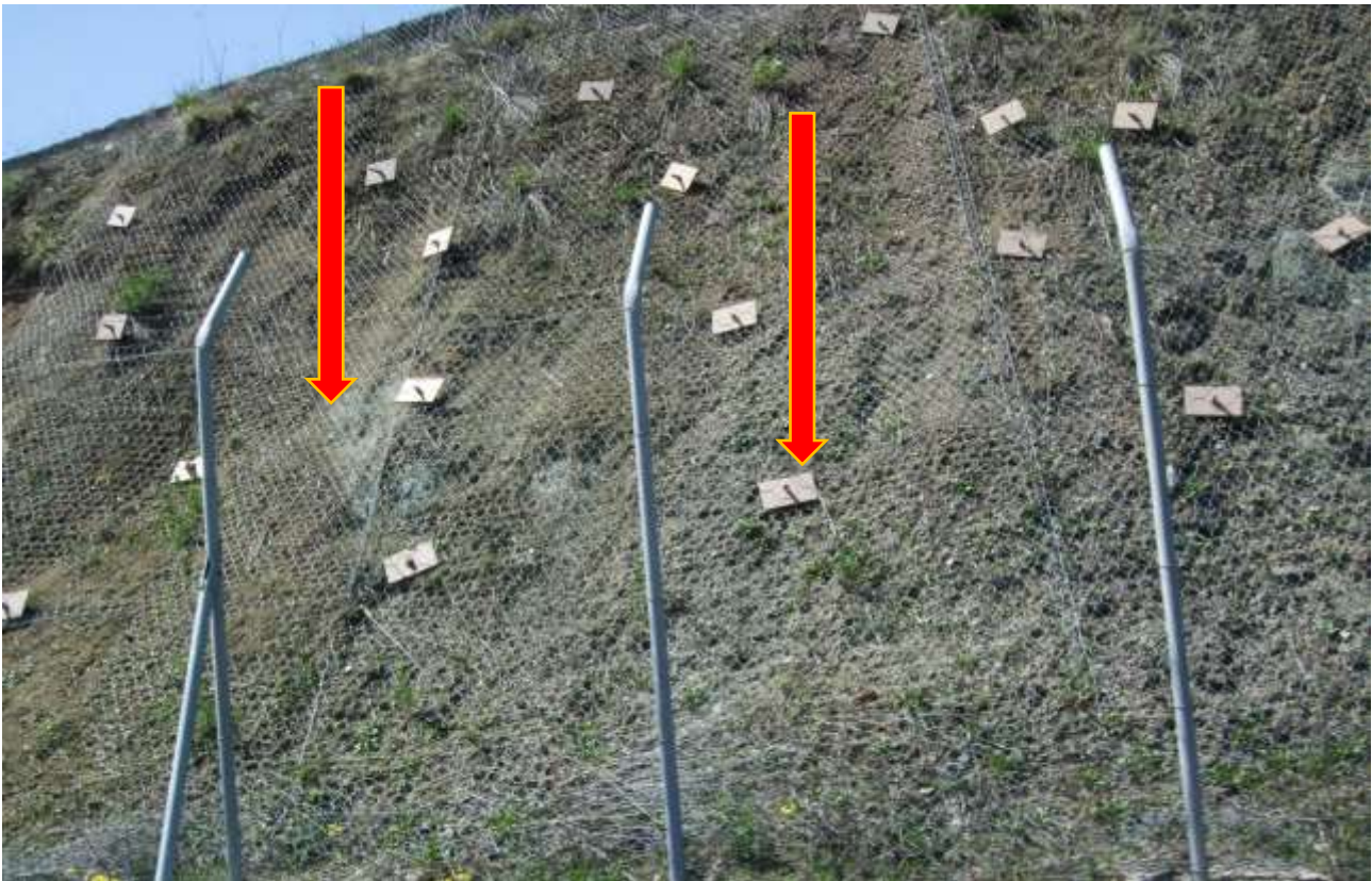
Figure A8.31: The dam slope has been fastened with anchors and lining mesh
