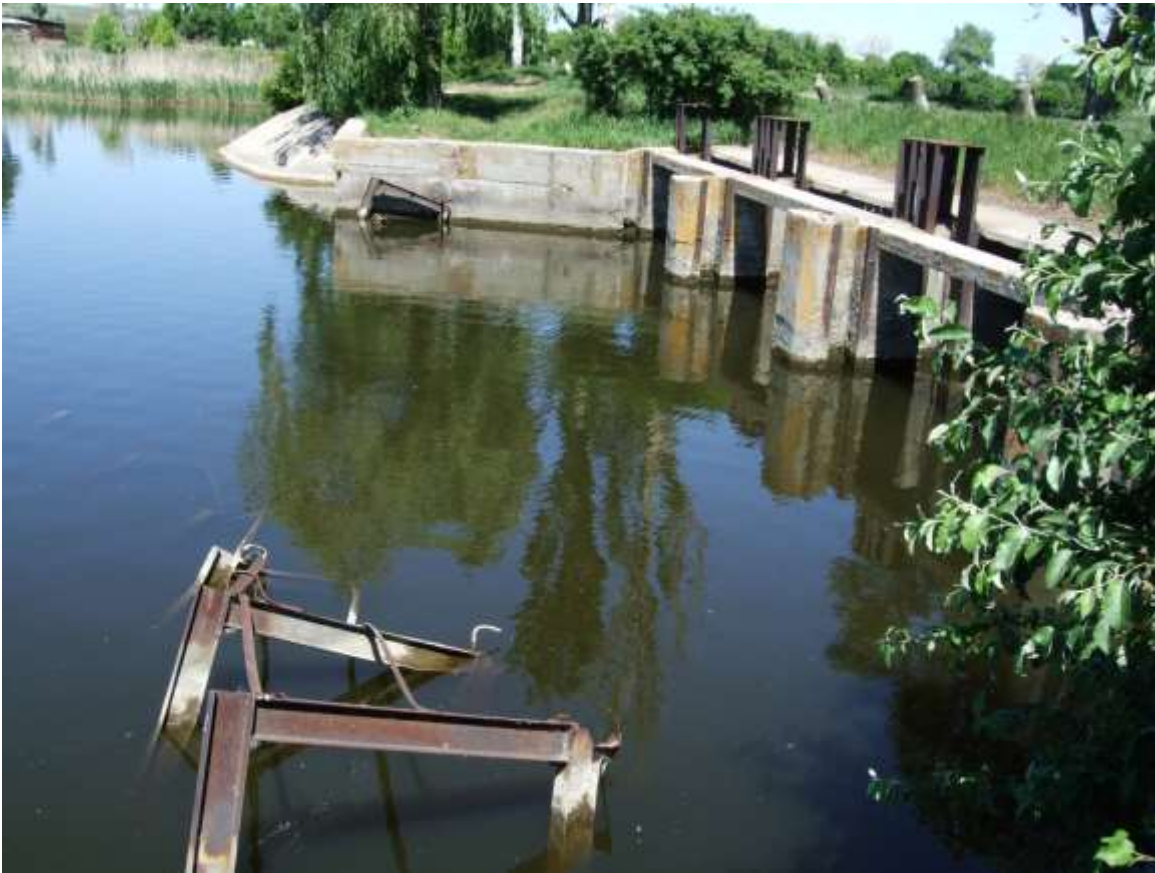
Figure A8.1: Spillway of tunnel type. Protective spillway grid is destroyed as a result of vandalism
