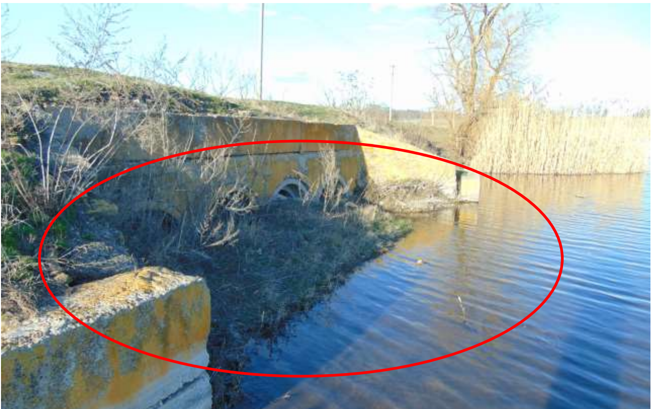
Figure A8.4: Emergency tailings spillway with the inlets blocked by sediments.
