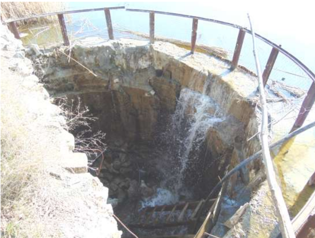
Figure A8.2: Spillway of mine type. Clogged shaft causes overflow through the dam
