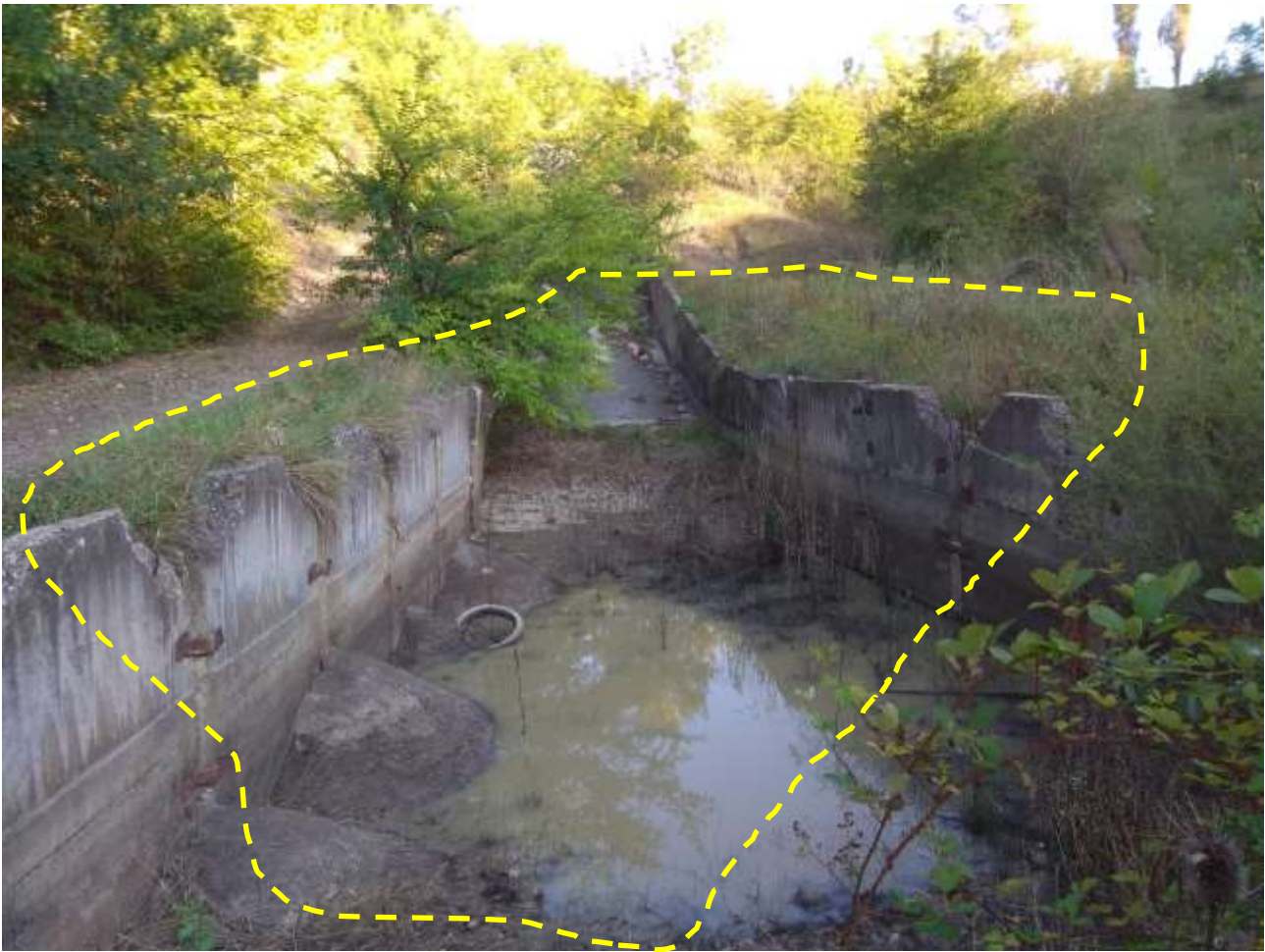
Figure A8.5: The clogged channel of the tailing pond prevents full water evacuation
