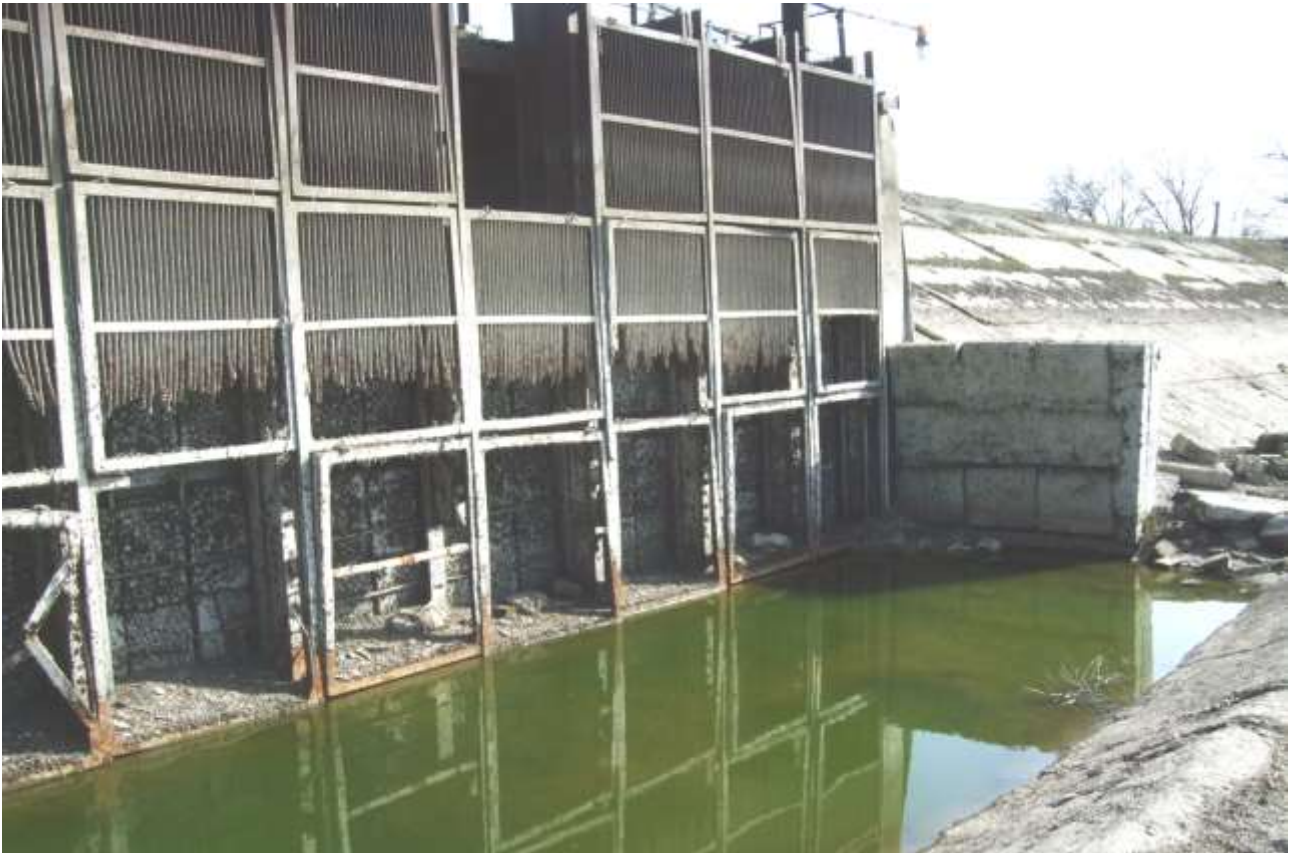
Figure A8.3: Spillway of mine type. Protective grid was destroyed by corrosion; as a result the spillway does not function.
